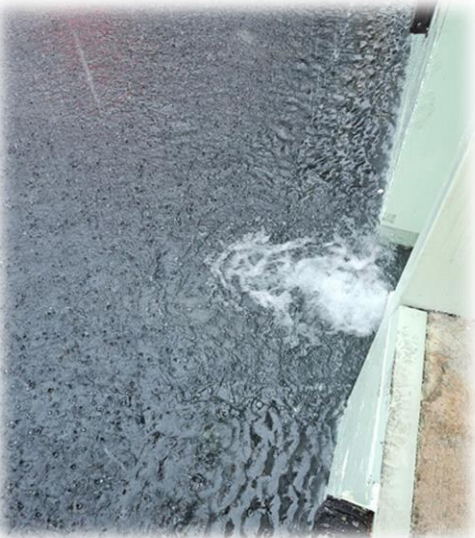
Water volume from the roof's downspouts into the overflowed parking lot drains!!
