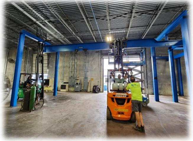
Securing the over 30' straight beam while the supports are removed/torched off for disassembly
